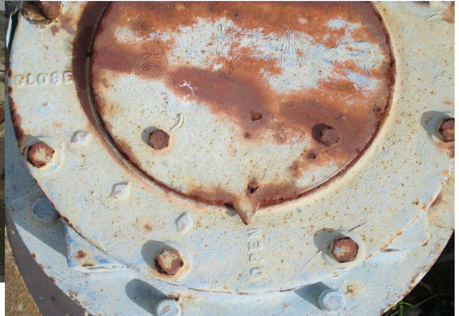
Valve in Open Position
