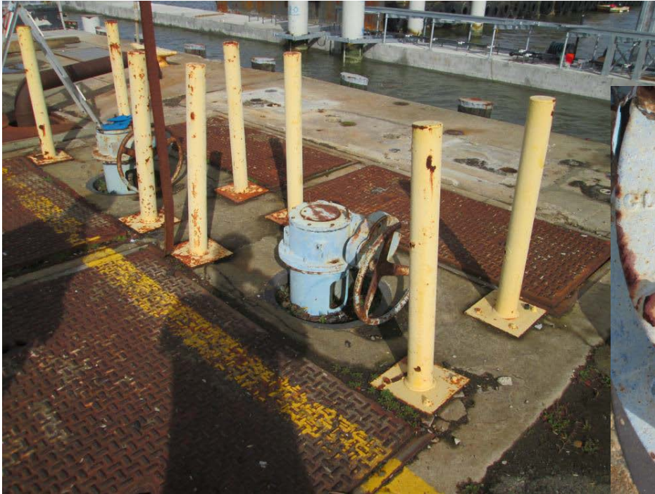
CWL-IA Valves at Mare Island Strait
